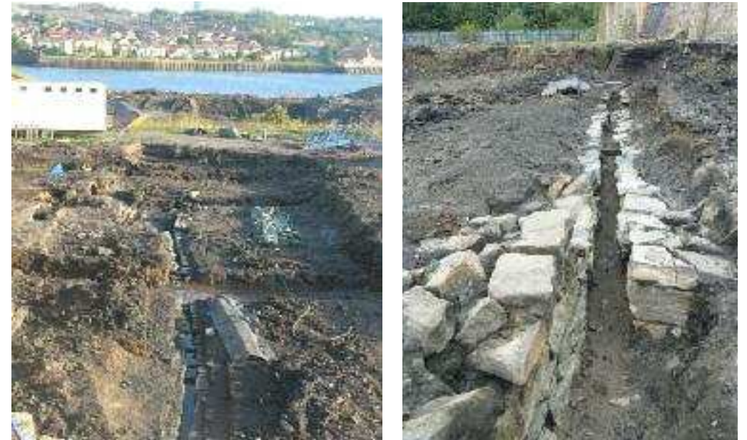
65 View of the course of the leet from the north, with capping removed.
